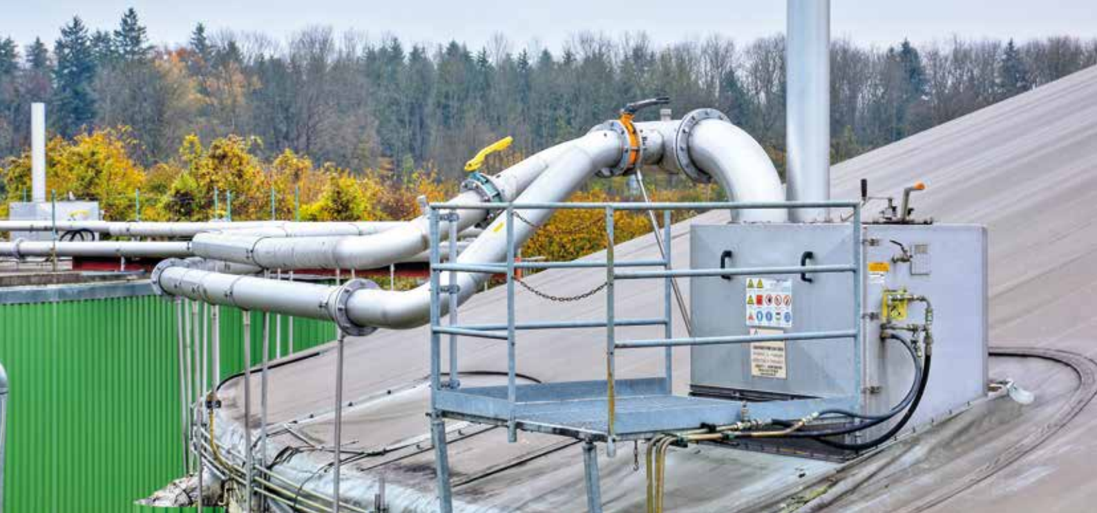
First generation of service-box in operation for over 20 years
