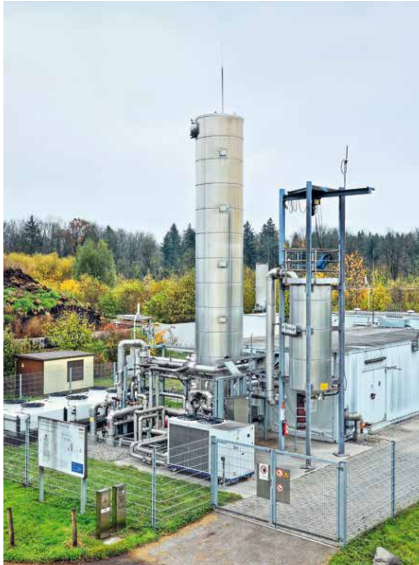
Gas processing plant
