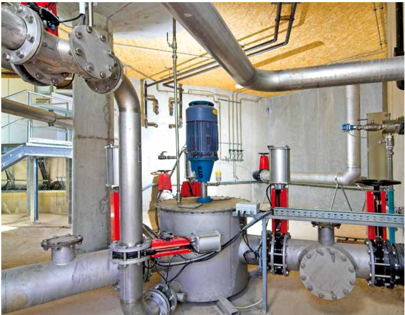
ZPS 4000 (central pumping station)
